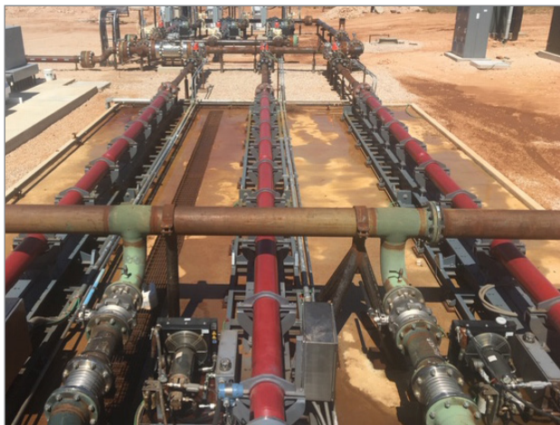
Each HPS unit meet unique requirements, including retrofit of existing pumps, and all programmed with automation controllers to efficiently move produced water to disposal.
