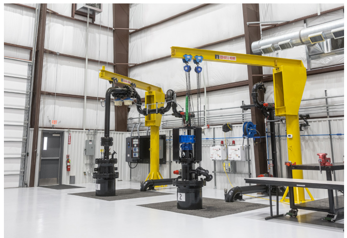
Summit ESP® Vertical Testing Facility located in Tulsa, Oklahoma combines experienced scientists and engineers with full system integration testing for all geothermal ESP systems.
