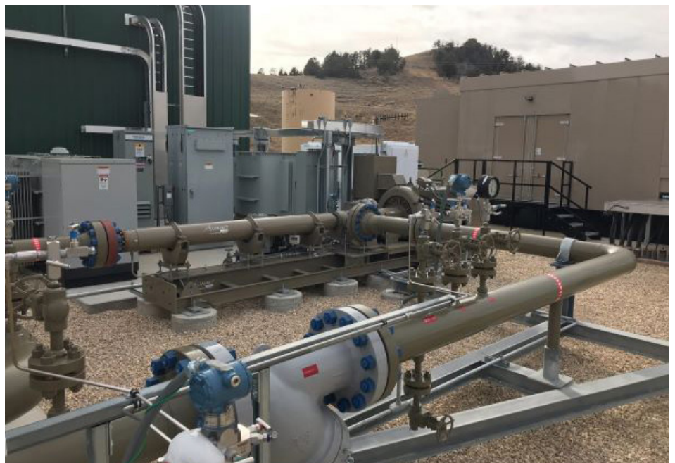
Summit ESP horizontal pumping system for injecting CO 2 .
