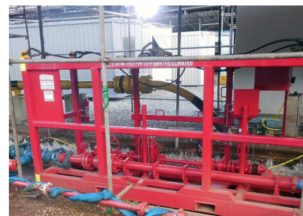
Remote pressure control discharge flow manifold at pig receiver location
