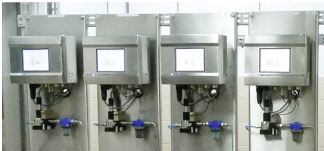
Oxygen sensors mounted on a panel in the water steam cycle
