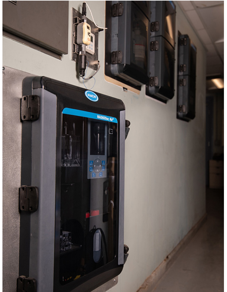
Fig 2: The Hach NA5600sc Sodium Analyzer
