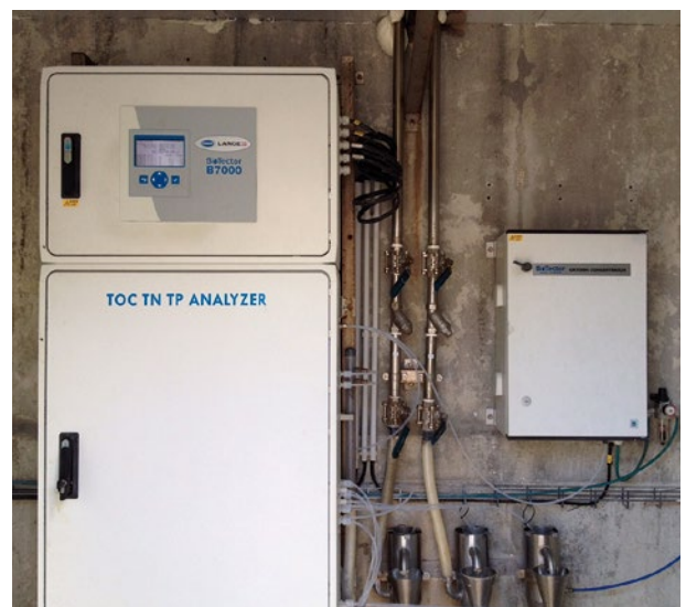
Fig. 1.: Installation of the Biotector B7000 in the analyser house
