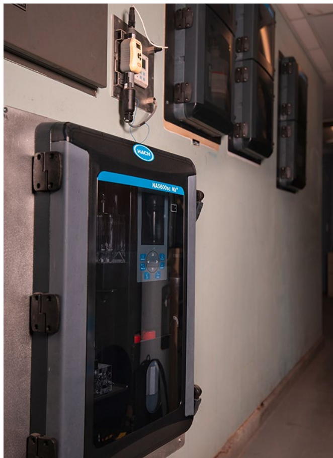
Figur 2: Hach NA5600sc natriumanalysator
