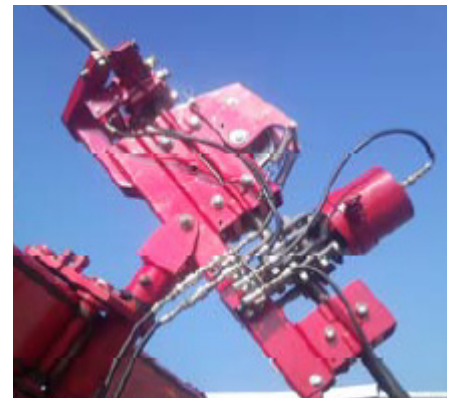
CT catenary head
