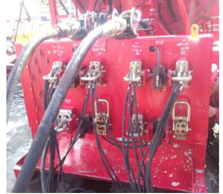
Catenary control panel
