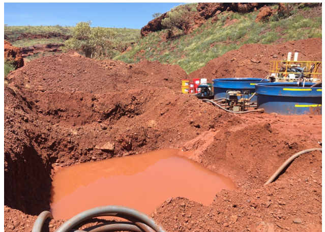
Limited space available for settling sump and tanks
