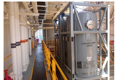
Figure 3. The BaraSolve™ Engineering Services team has installed the first two BaraStream™ HCB™ tanks (at right).
