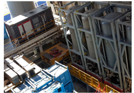
Figure 2. Four BaraStream™ HCB™ storage tanks are shown at right.
