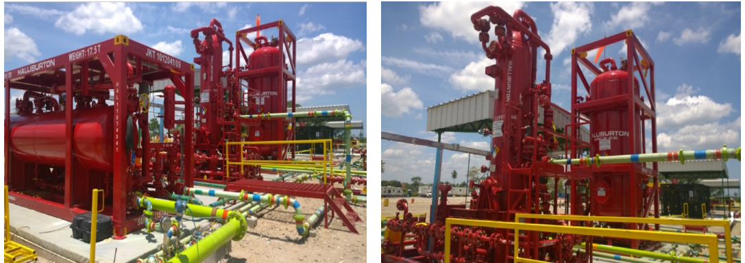
Close-ups of EPF equipment components in the Santuario 400 field, showing gas separators (left) and a rectifier (right).
