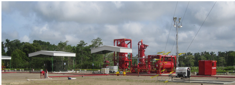
Photo of standalone EPF installation in Santuario 400 field
