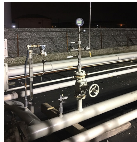
Ethylene Pipeline System
