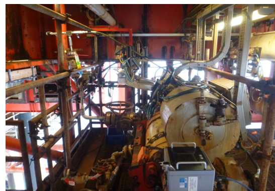
InnerVue™ PipeSuite datalogger connected to the system.
