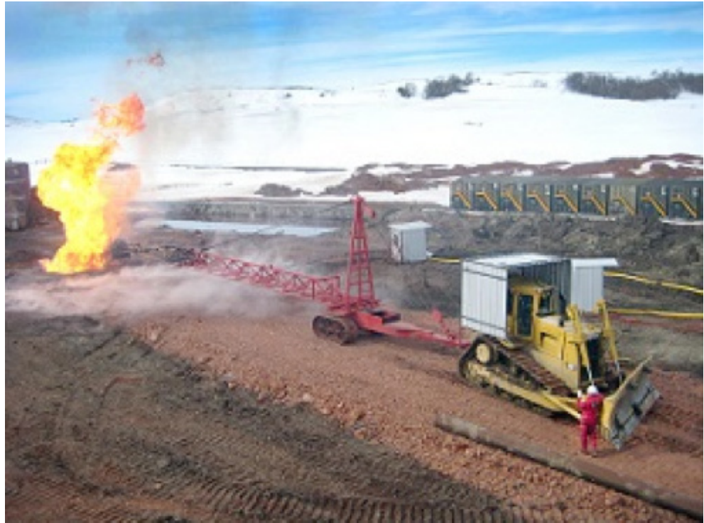
Figure 4. An Athey wagon is utilized in a well control operation. It is moved into place by a bulldozer that uses corrugated tin to protect personnel and equipment from the extreme heat of the oilwell fire.
