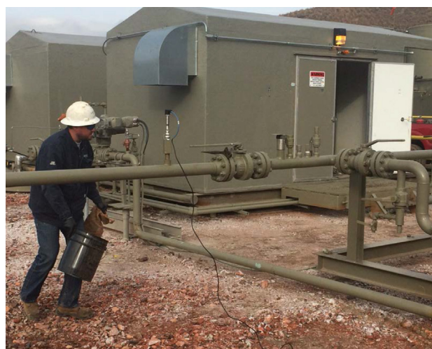
Figure 1. Shows high-resolution pressure transmitter tied in to the customer’s pipeline system, with an operator ready to operate the valve.
