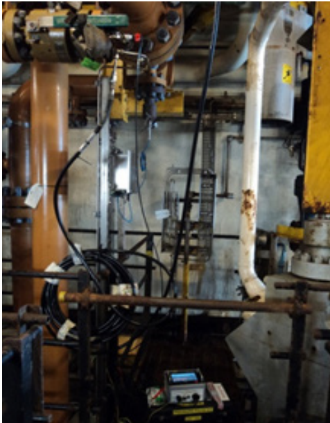
InnerVue™ PipeSuite survey equipment connected to the pipeline via instrument point.
